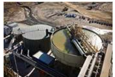
Lithium Recovery Plant
