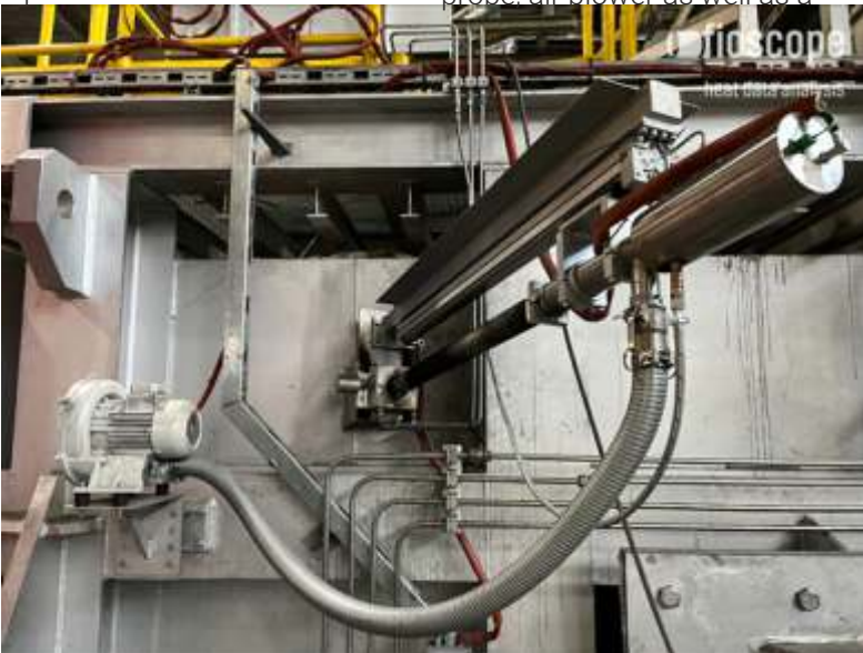
Figure 2: Fioscope Camera Probe and Air-Blower Mounted to Furnace Side Wall.
