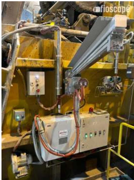
Figure 3: Fioscope Retractable Camera Probe and Air-Blower Mounted to Furnace Side Wall.
